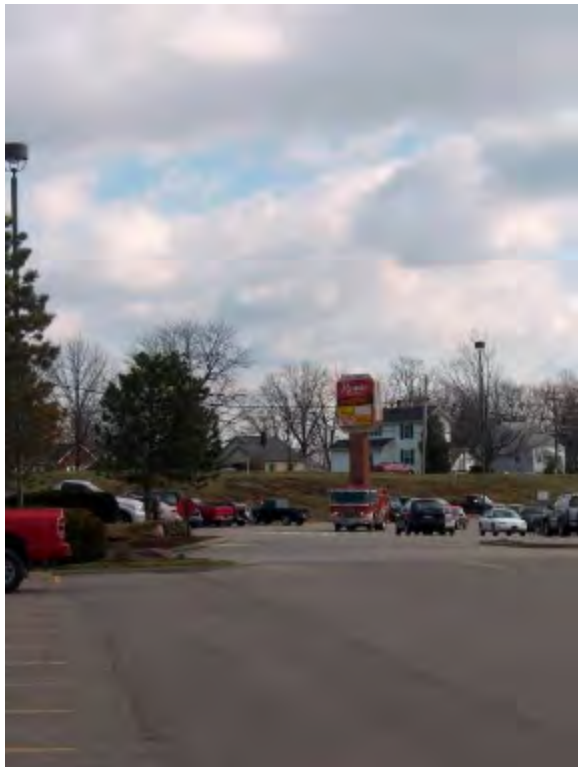
Land Slippage at The Shoppes at Taylor Mill Parking Lot. Source: Woolpert, Inc. 2006
