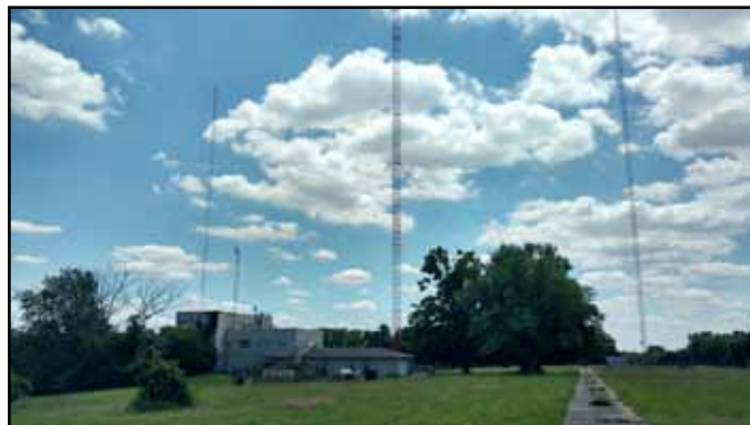
Figure 3.16 - WCKY AM radio transmitting facility
